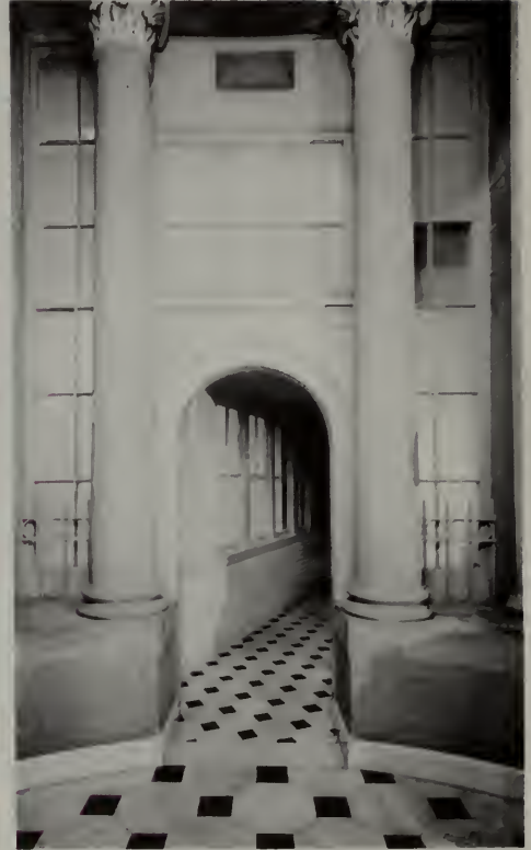
Second floor passageway before reconstruction. The passage was constructed in 1901. At that time, the walls were covered in white glazed brick.
